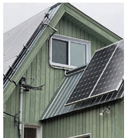
LANARK SOLAR POWERED OFFICE © COURTESY OF PLENTY CANADA
